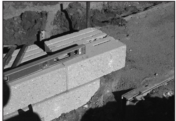
8. Step up leveling pad and base course in 6-inch increments when grade changes.
